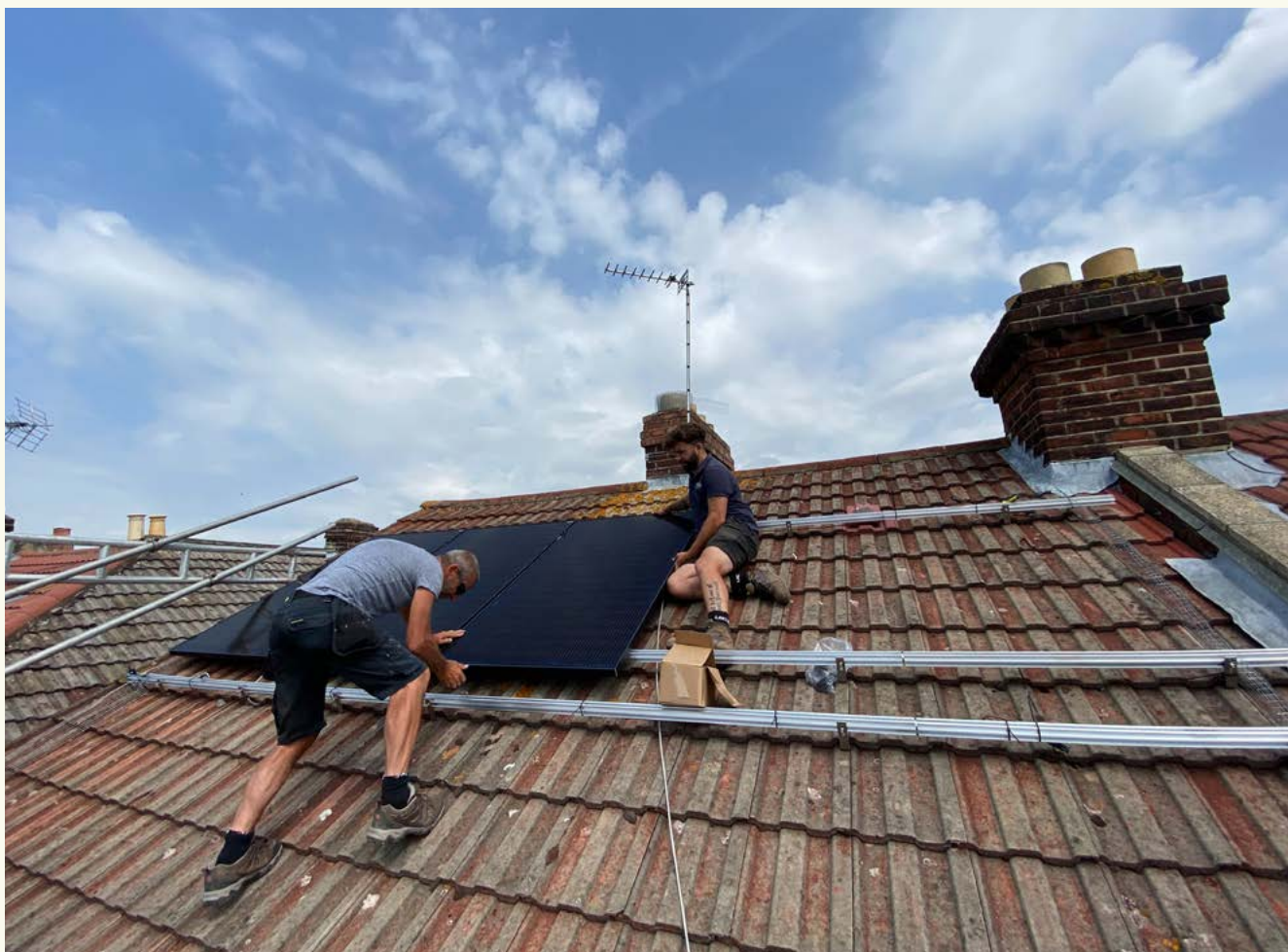
▲ Image of solar panels being installed in Portsmouth – part of the Switched on Portsmouth project
